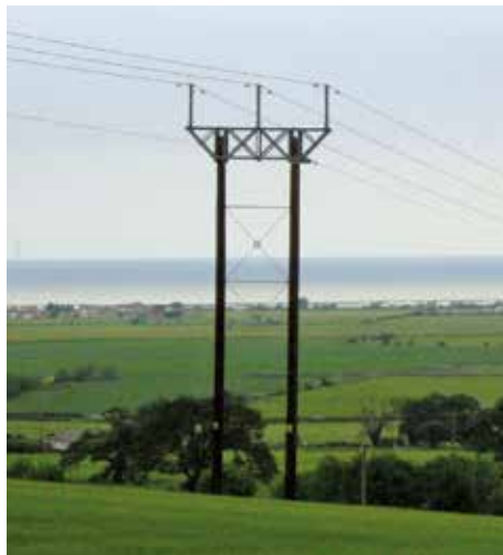
Heavy duty double wood poles – approx. 15m
