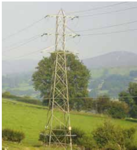
Steel pylons – approx. 26m
